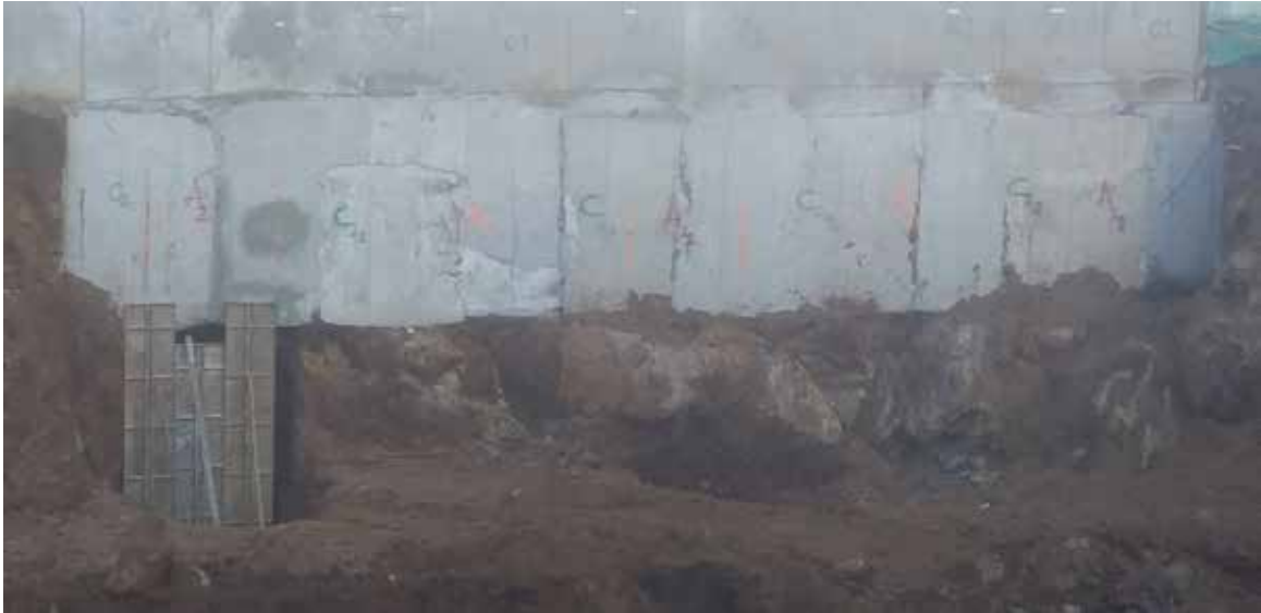
Photo 6: Setting out for second set of underpinning and shuttering to A2 pin.
