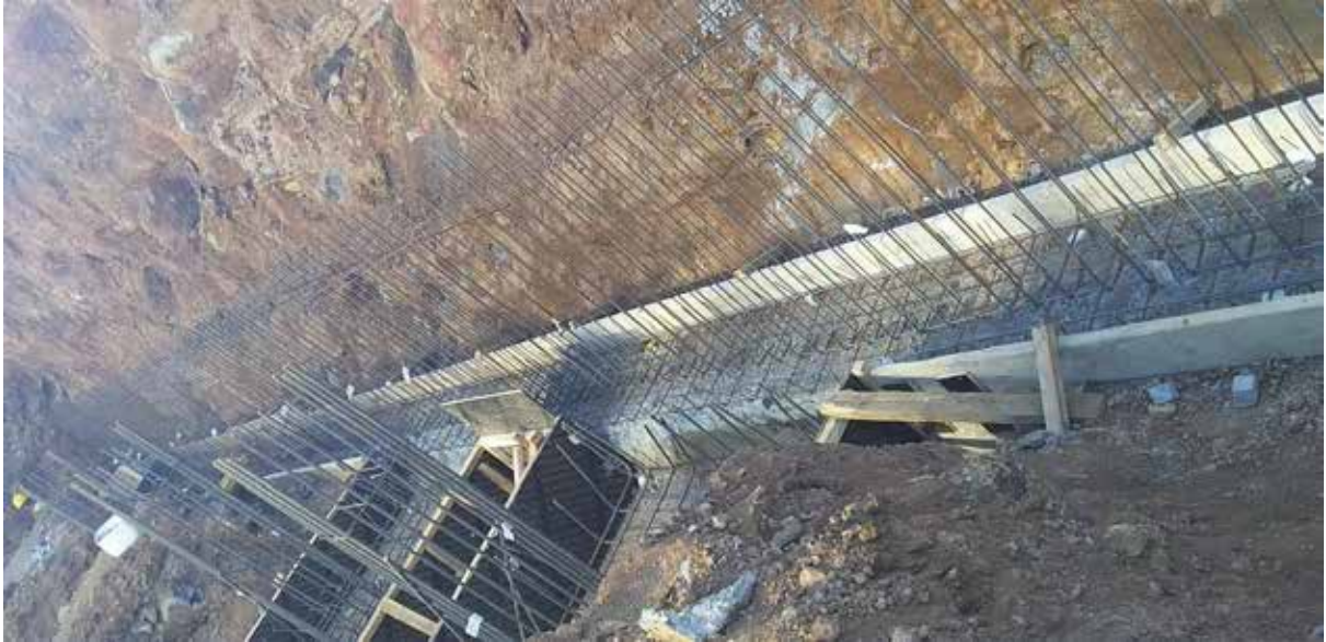
Photo 4: Formwork and Reinforcement to retaining wall base and starter bars for retaining wall along GL 7'/E-K'
