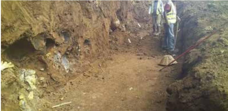
Photo 1: Trimming & Compaction for retaining wall base along GL A'/1-7' prior to blinding.
