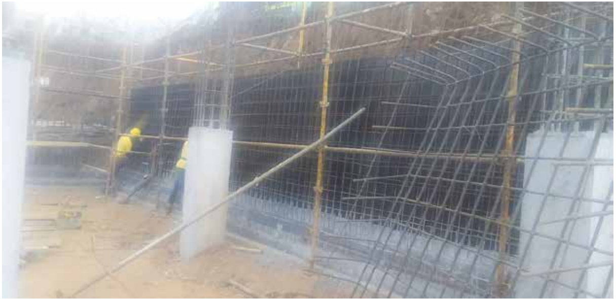
Photo 8: Reinforcement & Shuttering to 2 nd lift retaining wall (below soffit of B2 slab) along GL F-J/7'
