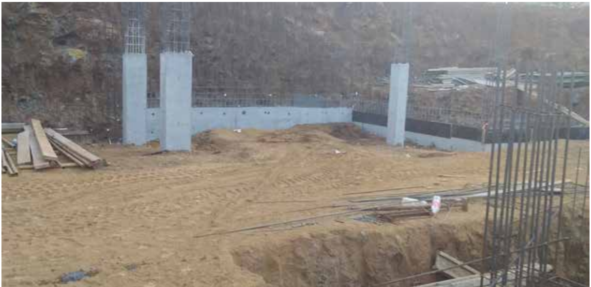
Photo 10: Casting of column and retaining wall and selected fill between GL J-K'/1-7'
