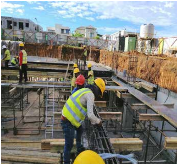
Photo 11: Reinforcement and formwork to beam at soffit of Basement B1 along GL E-J/5
