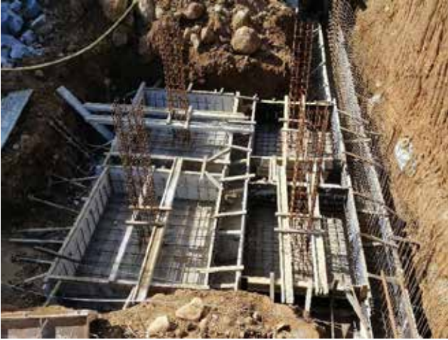
Photo 13: Shuttering to reinforcement of column bases along GL B-C|5-6 and strip footing along GL Ax'-D|6
