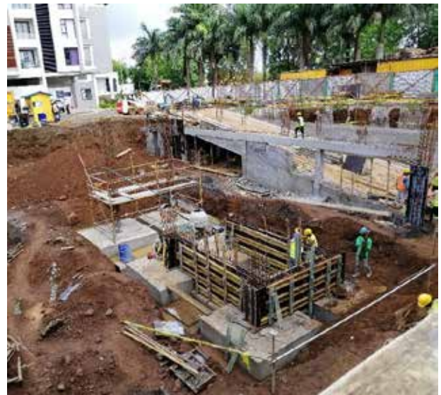
Photo 8: Formwork and reinforcement at retaining wall of staircase along GL B-C|1-2 and column at GL B-3 and GL C-3
