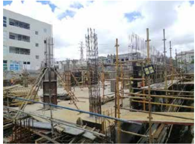
Photo 14: Shuttering to reinforcement at Lift Pit, columns and retaining wall along GL E'-J|7 at Basement B1
