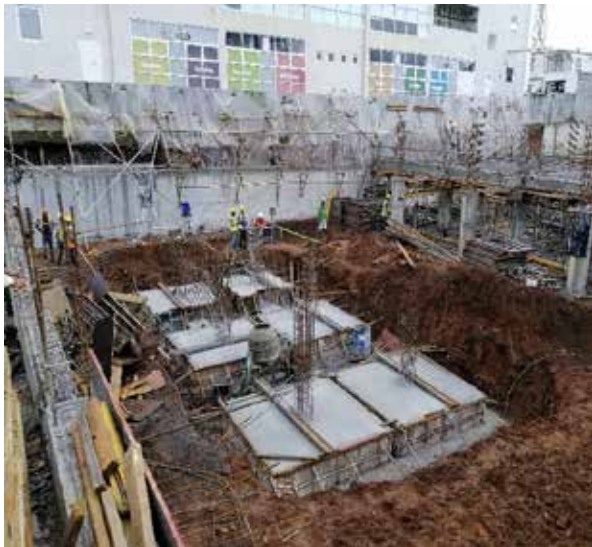
Photo 7: Casting of column bases and strip footing of retaining wall along GL B-C|1-3
