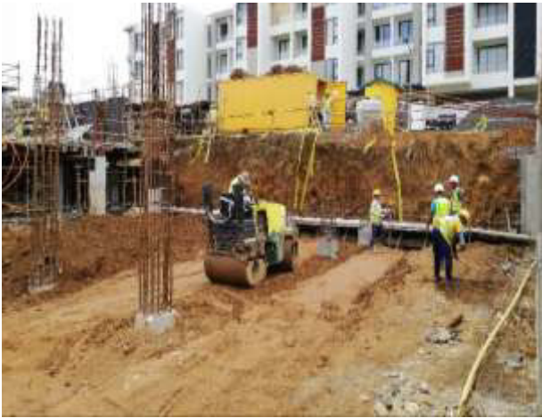
Photo 1: Soil Compaction along GL Ax-D|1-7'
